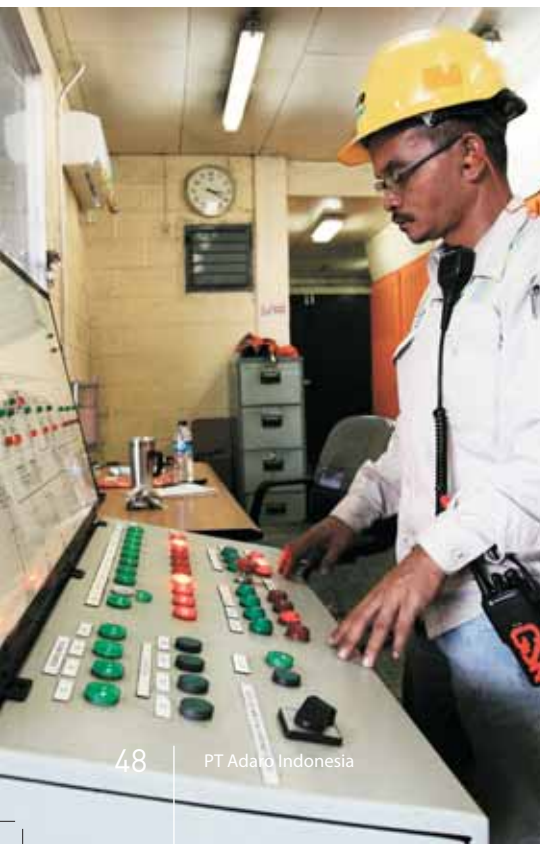
Left: Operator is observing generators through control panel in Kelanis
